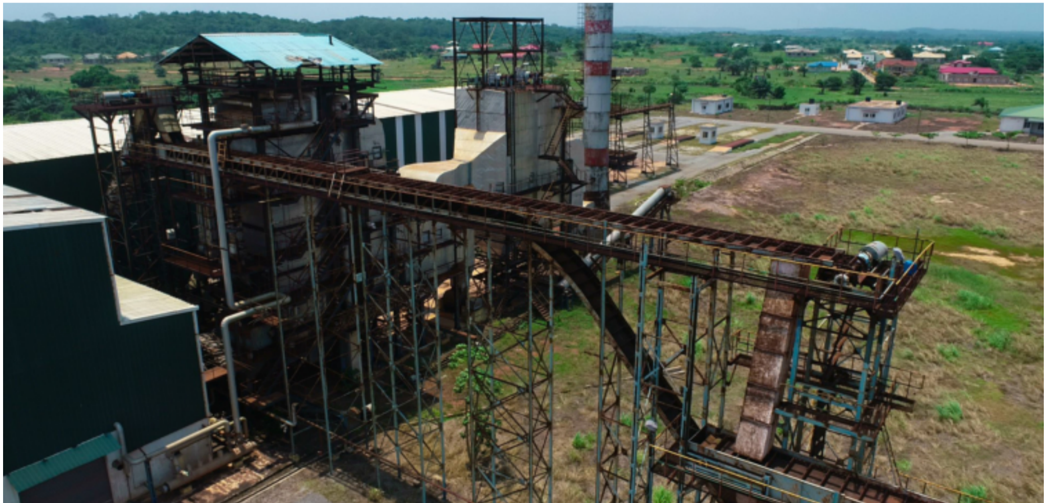
The Komenda Sugar Factory has failed to produce sugar and is currently rusting away after six years of commissioning.
